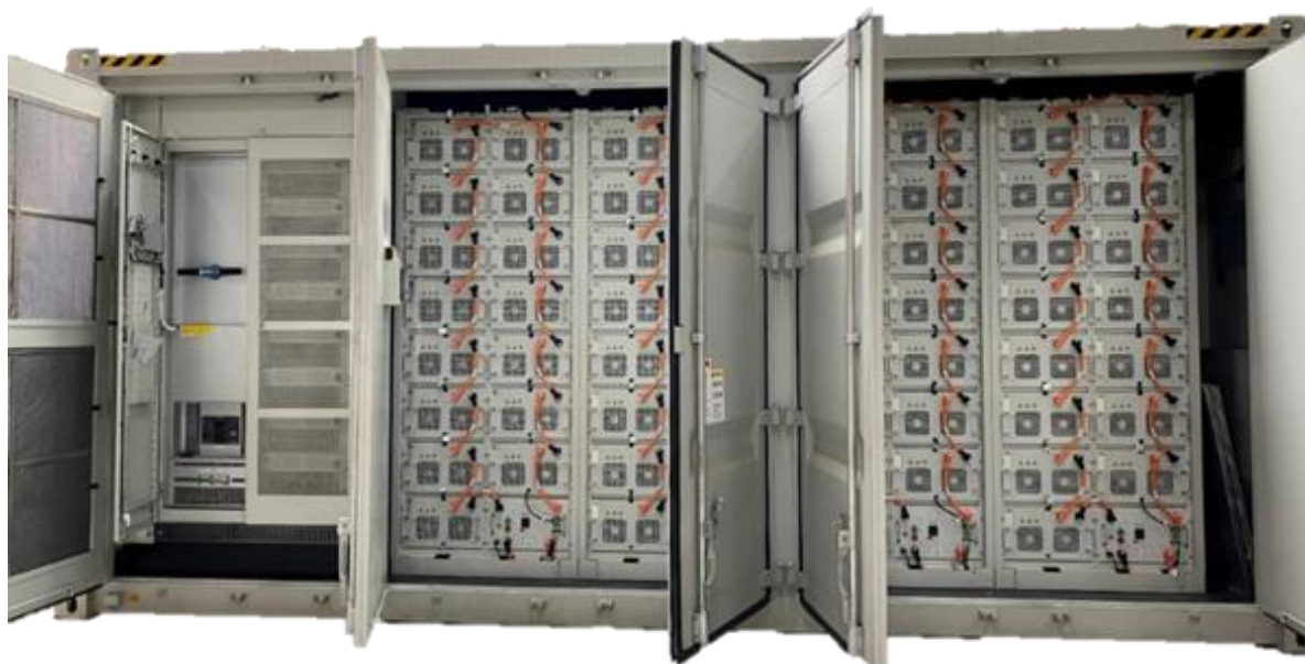
Figure 2 – Battery Energy Storage System
